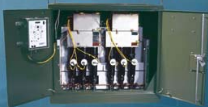
Automatic Source Transfer Package
